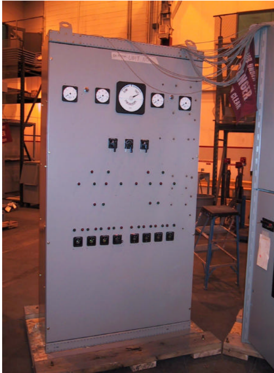
Example of a panel currently under manufacture, for remote breaker controls, furnished by Burlington.
